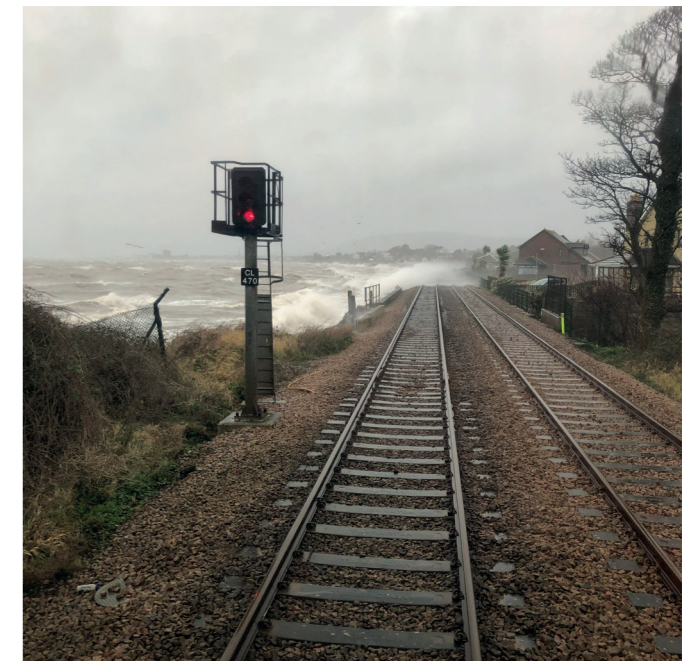
Storm impact, Downshire (Larne railway line) Image courtesy of Translink
