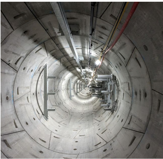
LPT2 tunnel completed, with bracketry installed ready for the cables to be pulled in and fixed.
