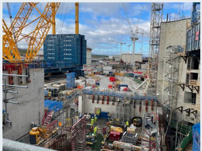
Crayford slabs on a pit bottom HK Fuel building under construction at HPC (reactor building is to right of image).
