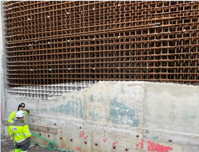
Wall 206 after shutter leak occurred
