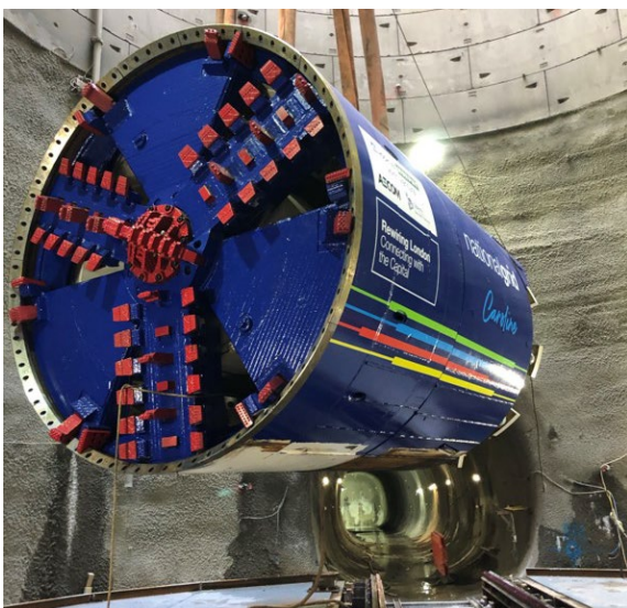
LPT2 - Tunnel Boring Machine (TBM) dropped down the shaft in preparation for the TBM launch.
